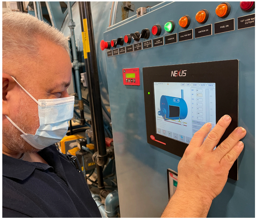
Boiler Plant Operator Dennis Aldrich removes the boiler from “hot standby” during a heating redundancy check at Manchester VA Medical Center.
