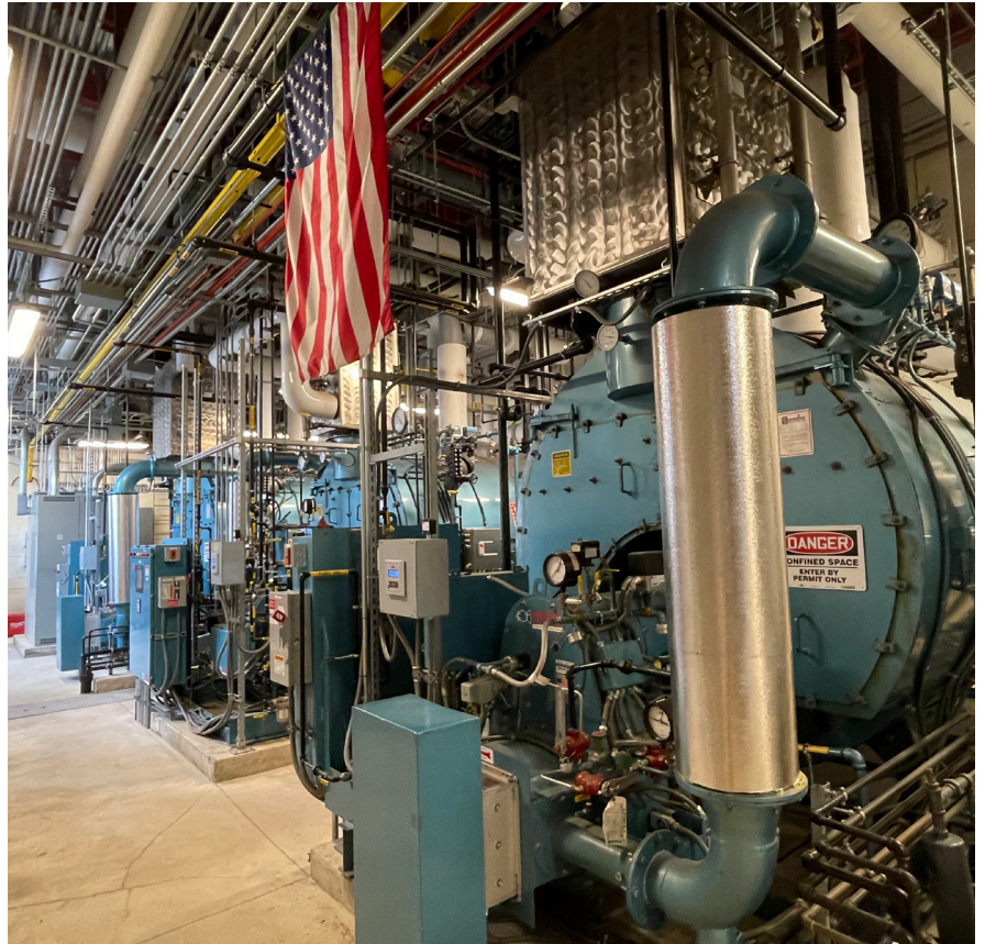
The Manchester VA Medical Center boiler plant enables heat, hot water, and equipment sterilization for patients and staff utilizing the facility.
